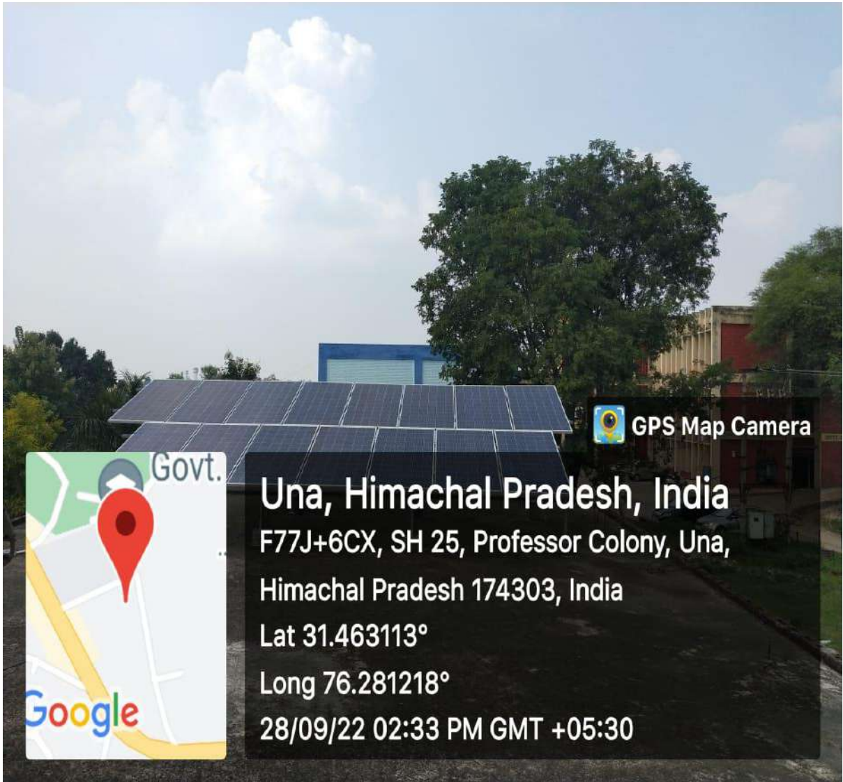
Figure 13 Grid connected Rooftop solar power Plant.
