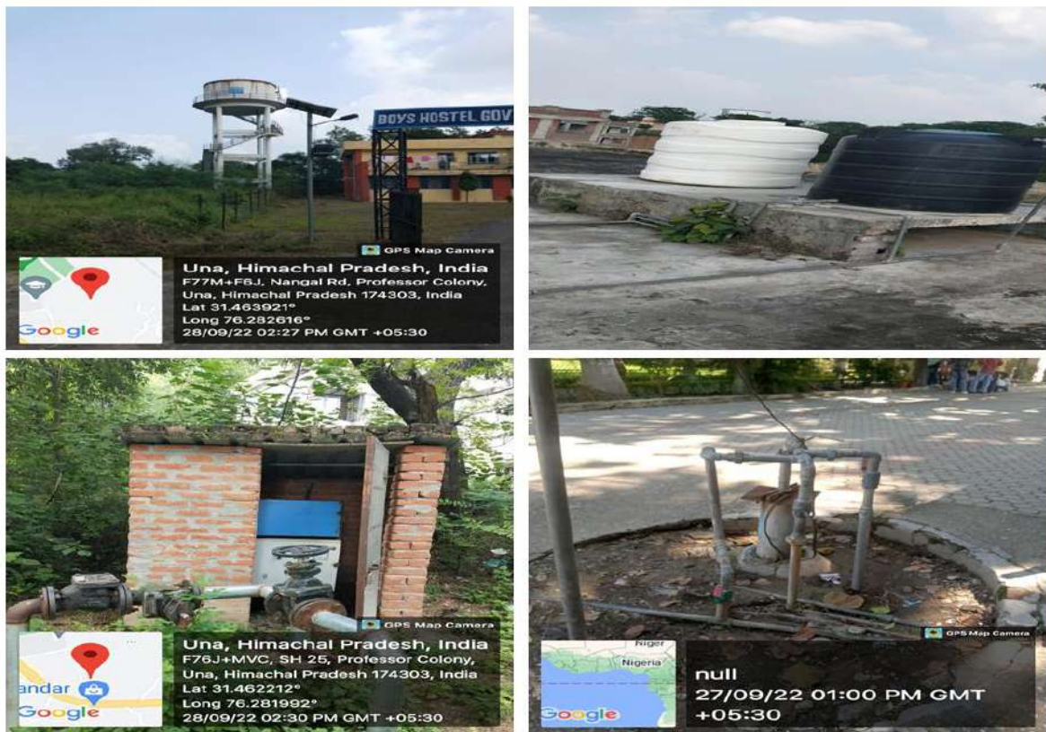
Figure 8 Water Storage in Tanks , distribution and control system for proper water supply.
