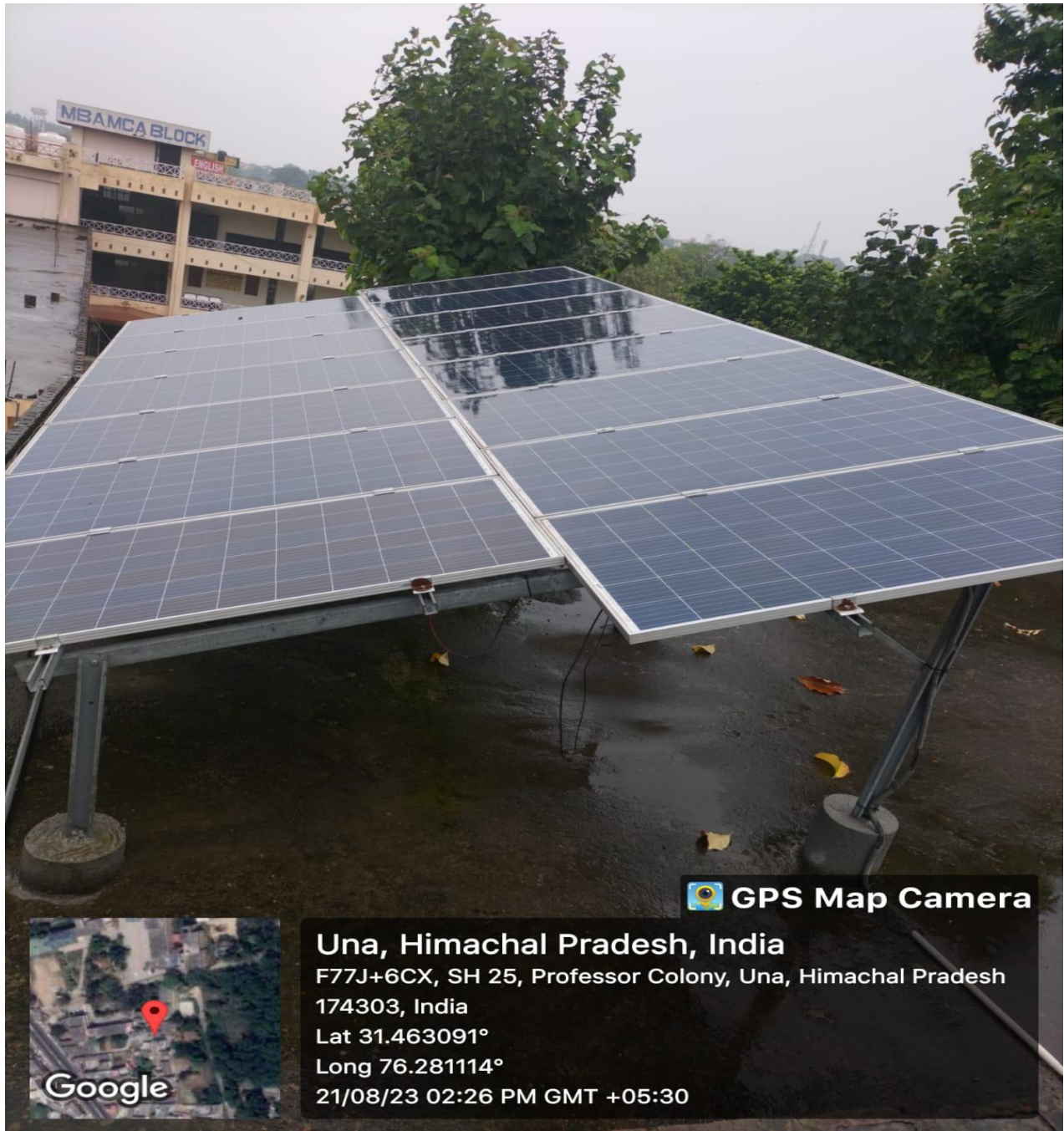
Solar grid installed on the roof of the BCA department.
